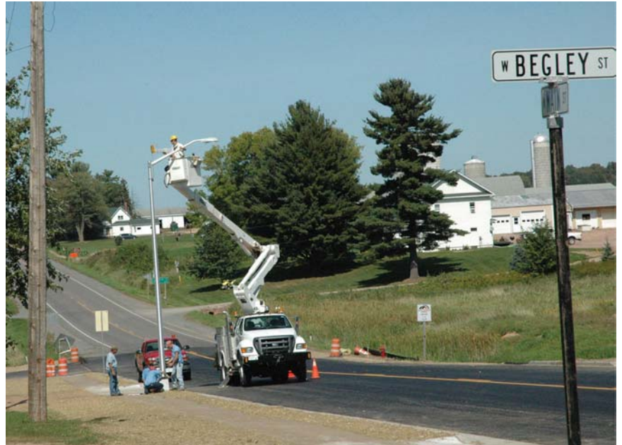
Clark Electric crews help the City of Greenwood install the final street lights on the north side of town.
