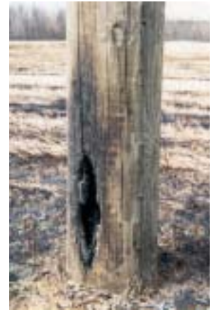
After a small ditch fire, this pole will need to be replaced.
